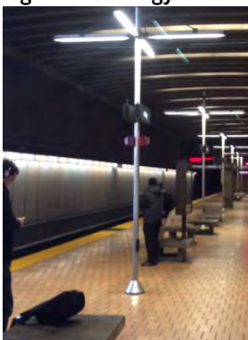
LED replaced fluorescent lighting at Ashby BART Station
