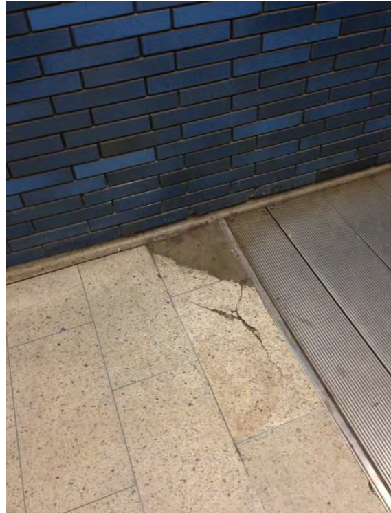
Floor in need of refurbishment
