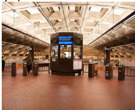
LED fixtures in the Washington Metro have improved light levels and quality Source: http://planitmetro.com
